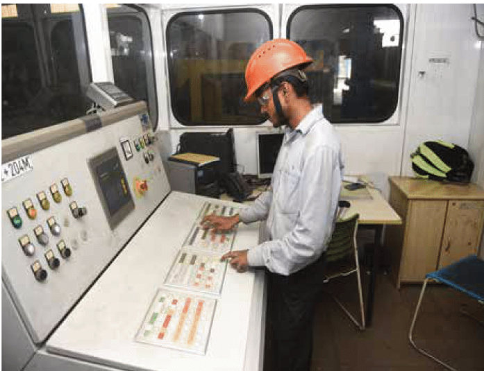
▲ The control room at the cast house.
